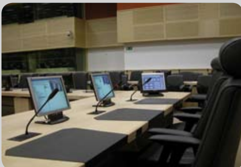
A flush mounted conference microphone with built in loudspeaker is installed at every seat
